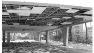
The damage to the parking area was the most visible.
